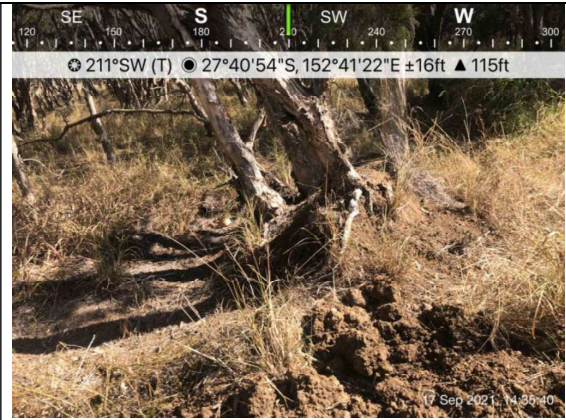
Figure 11: Soil from the stockpile area beginning to impacted on roots
