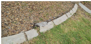
Concrete continuous edging is cracked and grass growing through
