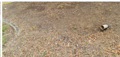
Drain pipe through garden bed (out pipe)- invites erosion, no filtration by rock or planting, unsightly
