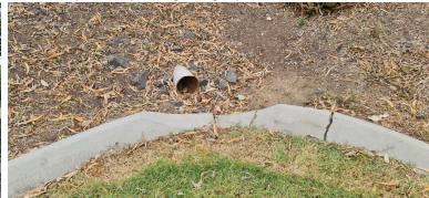
Drain pipe (in-take) looks too high for capturing water, possible poison is being used to control edging which will contaminate nearby river
