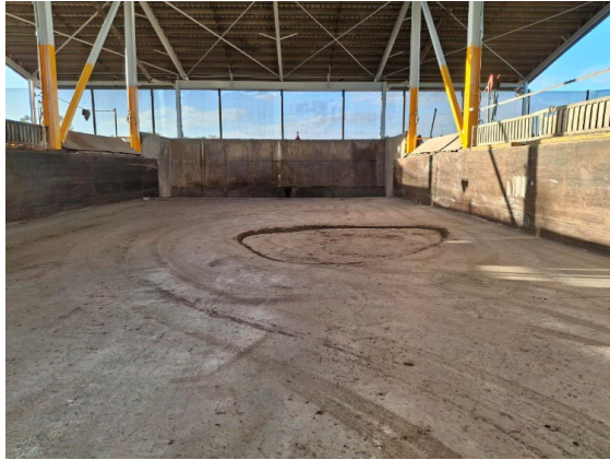
Pit floor topping slab delamination area.
