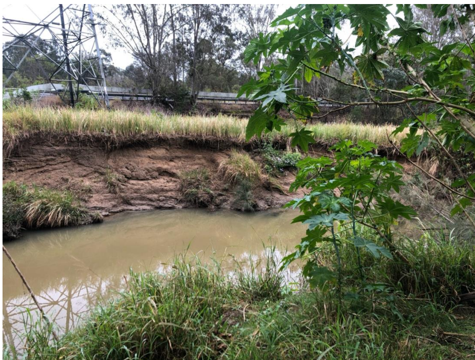
Figure 2 Site BU002 showing continuing erosion under powerline.
